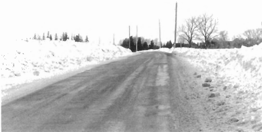
Figure 7. Snow Accumulation Along Woolwich Street Without Snow Fences
