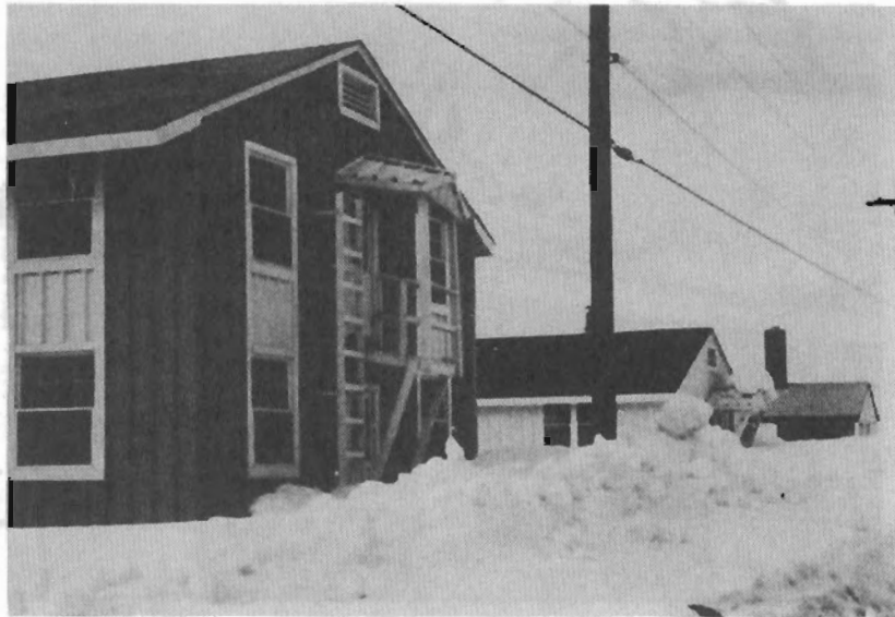
Figure 5 Collapse of Lower Level Roof
