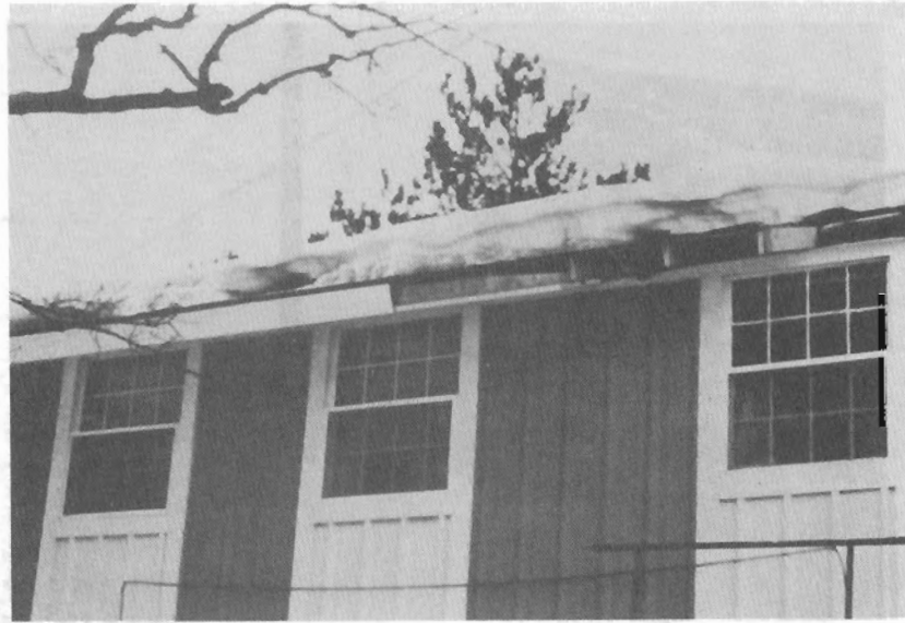
Figure 3 Partial Collapse Due to Eave Icing
