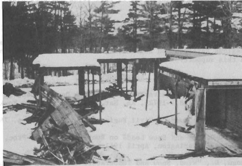
Figure 4 Collapsed Vehicle Shed at Fort Drum
